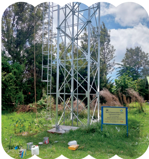
6m steel tower
