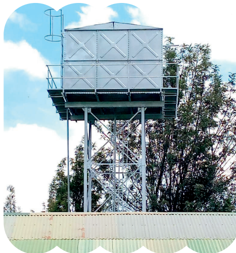
24m 3 prestressed steel tank
