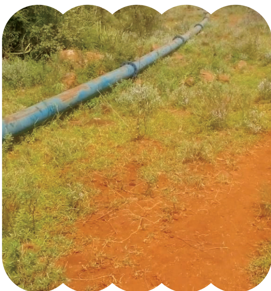
Conveyance line of GI 250mm
